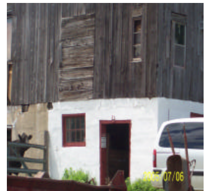
Fig 3: Old entrances and windows covered up
